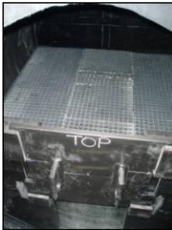
Figure 1. Removable bulkhead door across from ingress/egress ladder at rear of filtration chamber.
